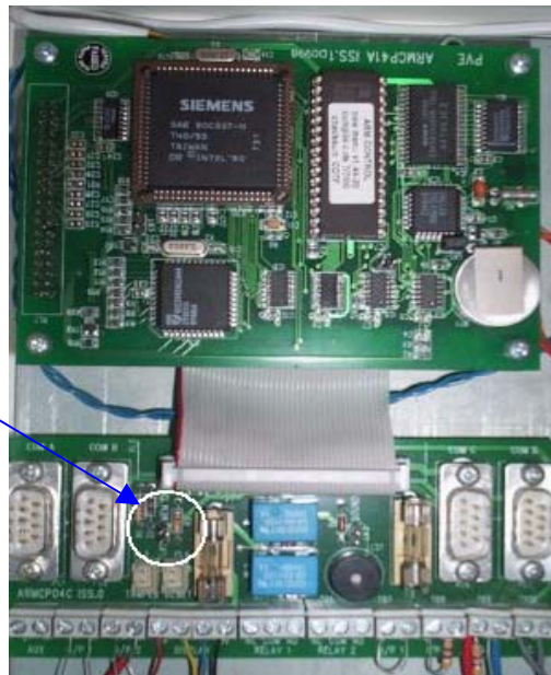
Control Panel PCB
